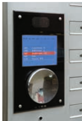
La Fenêtre has fire and burglar alarms, automated access control systems and a visitor registration system. The car park is monitored by CCTV. The service manager plays a significant role in service to residents
